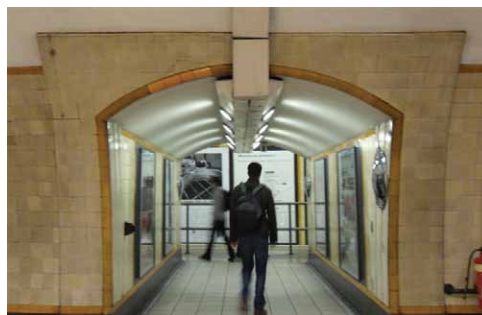
Fig. 2: Patch repair at Turnpike Lane around concourse entrance to platform. Note new bright yellow tiles on the entrance surround (author's photo).
