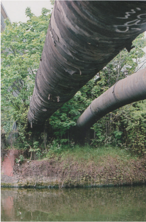
Figure 2: Pipes of the Northern Outfall Sewer cross the Lea Navigation. Photograph: J. Gardner.
