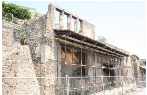
Fig. 15: Conservation work and the resulting barriers can have a negative impact on the visitors perceptions of the site if not properly explained.
