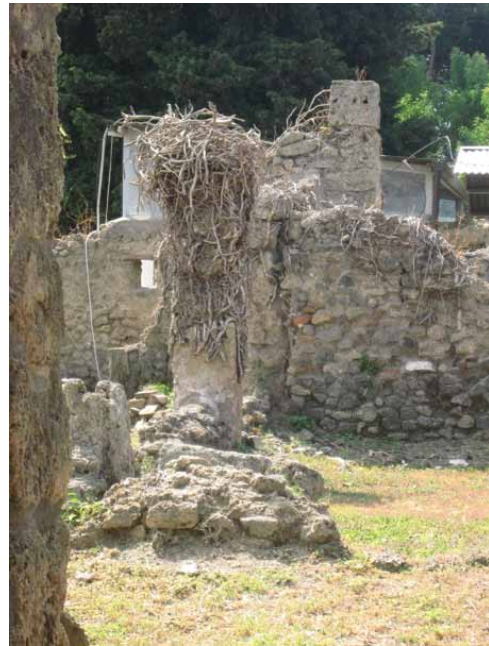
Fig. 9: Overgrown vegetation and crumbling walls in an unvisited area of site (area 15 in Figure 5).
