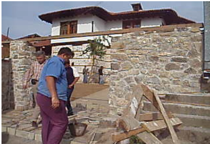
Figure 3. Cultural Heritage without Border's restoration of an Ottoman Town House in a Serbian Village 2006.
